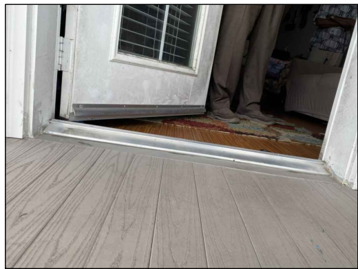
7 PHOTO @ OUTSIDE BALCONY DOOR BOTTOM A-143 N.T.S.
