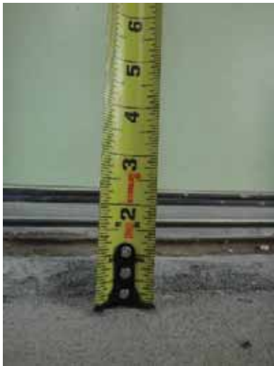
Threshold and change in level at primary entrance threshold exterior side, 1210 Rev. John Raphael Jr. Way.
