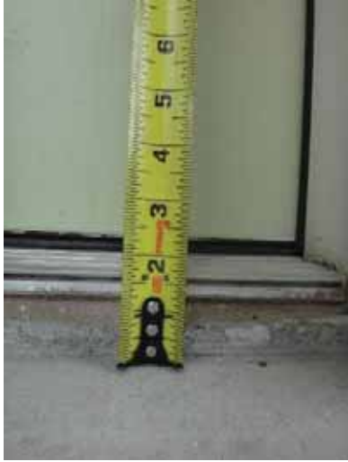
Threshold and change in level at primary entrance threshold exterior side, 1212 Rev. John Raphael Jr. Way.
